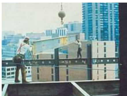
At-risk workers without appropriate safety equipment
